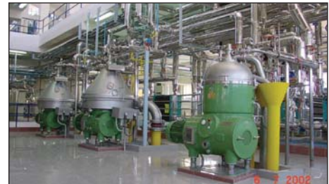
(i) A piping network in an industrial facility.
